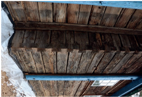
Figure 2. A view of the exposed log structure of the cemetery church of St. Onuphrius in Stryki, March 2023, author: Katarzyna Woszczenko
